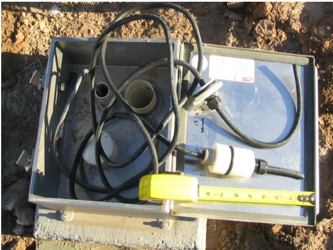
Figure 10 Photograph of packer (above measuring tape) used to seal pore-pressure transducer and cable in piezometer casings; transducer has yet to be attached to cable; photograph also shows fixtures at top of casing, including concrete pad, stainless steel protective box, piezometer casing, and electrical conduit (small casing through bottom of box) that leads to the instrument shelter
